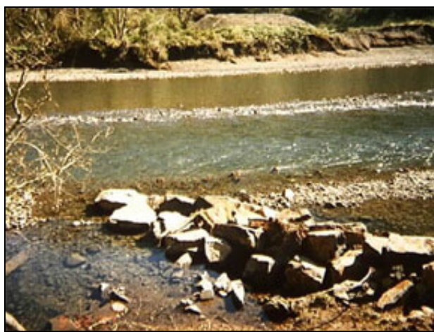
THIS recently completed barb is similar to the one constructed on Kevin Smith’s property. Barbs direct streamflow energy away from the banks
