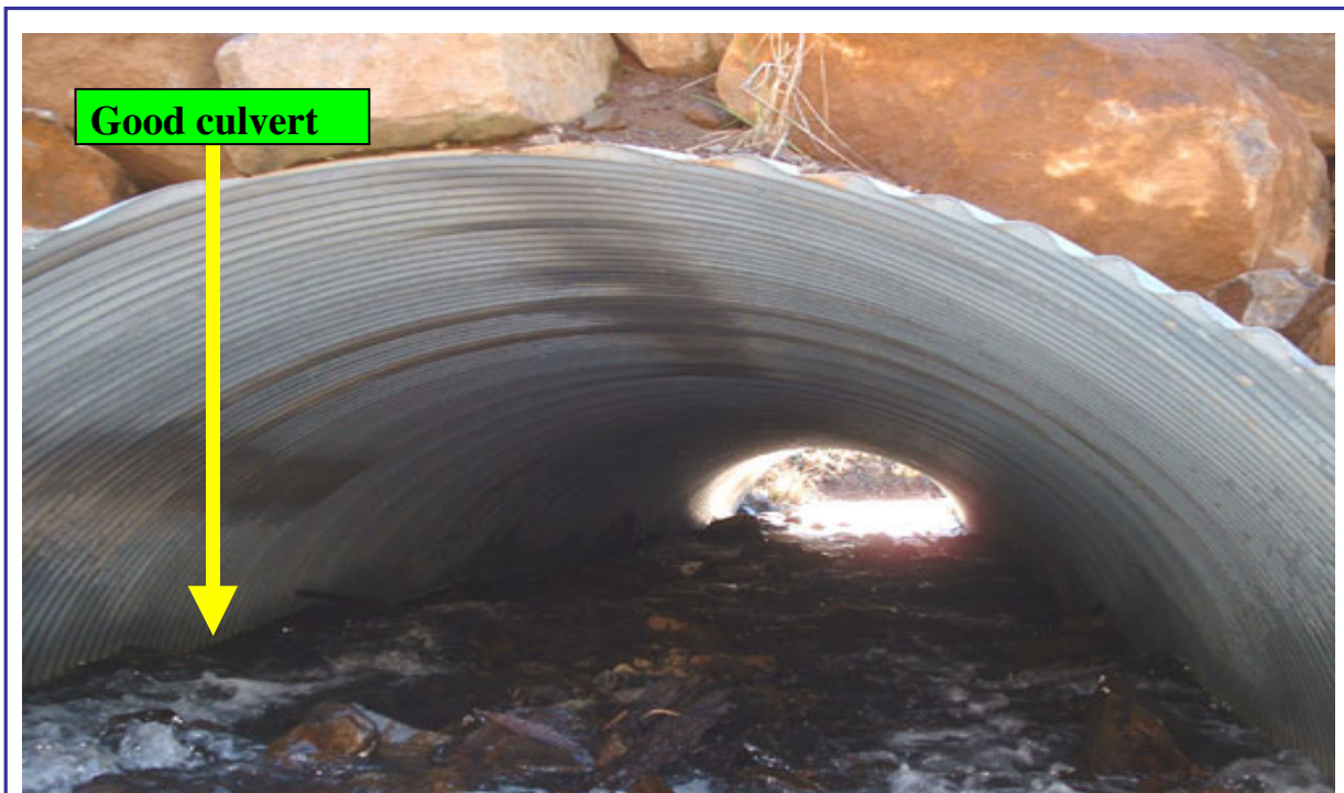
THIS culvert is level with the rest of stream and has lots of rocks and boulders, keeping the velocity of the stream consistent and allowing fish to easily pass through.
