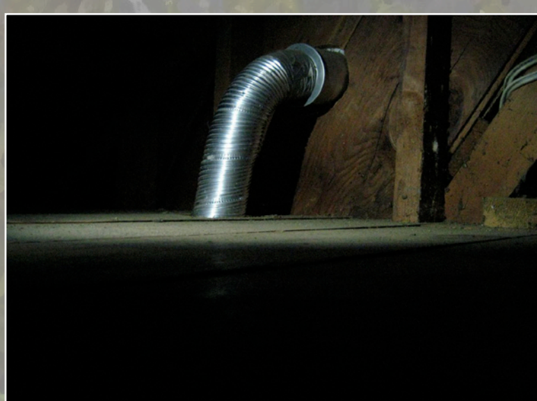
Vent fan ducting in attic
