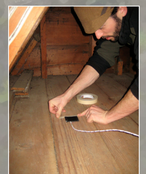
Heat Flux Transducer being installed above shower
