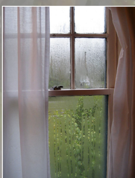
Bathroom window covered in condensation
