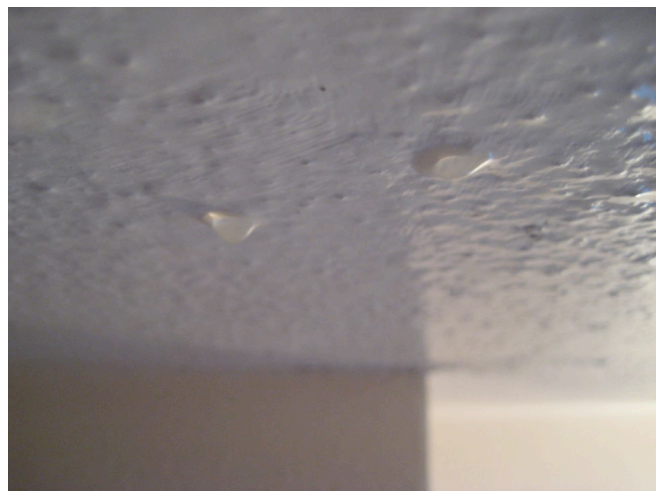
Fig. 7: Condensation on the bathroom ceiling
