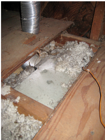
Fig. 9: Exposed insulation in the attic, showing some degradation
